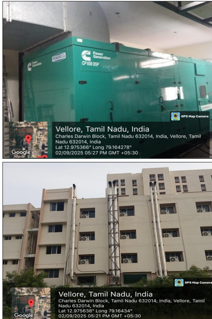
Figure 2.8 Photographs of DG sets with Stack
