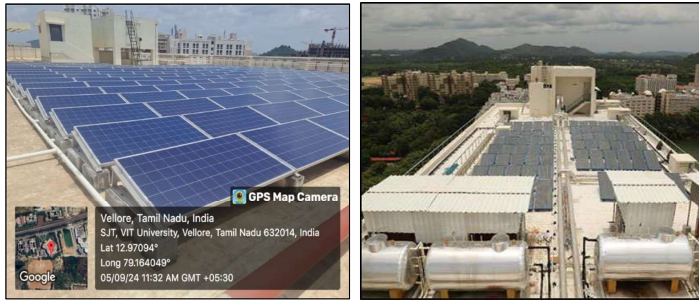
Figure 2.1 Photographs showing Solar Panels and Solar Water Heaters installed at rooftop
