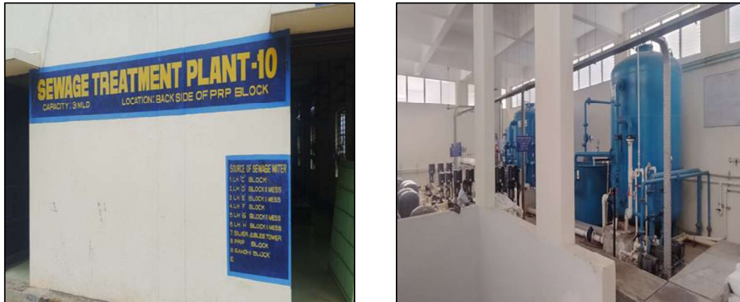
Figure 2.8: Photographs of the STP's installed within the premises.
