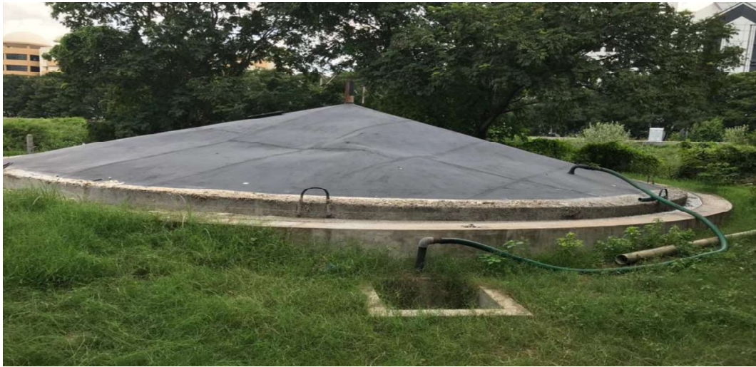
Figure 2.17: Photographs showing Biomethanation Plant
