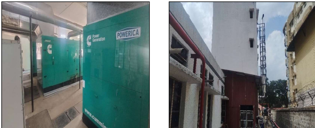
Figure 2.21: Photograph showing DG Sets provided with acoustic enclosure and stack height as per CPCB norms
