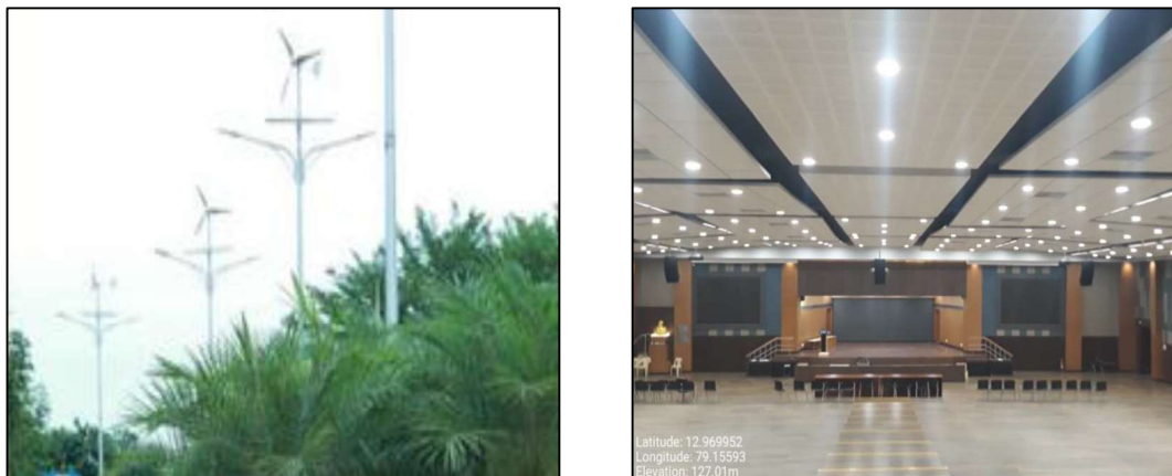
Figure 2.2 Photographs showing Solar and Wind Powered LED Street lights and LED lights provided in auditoriums
