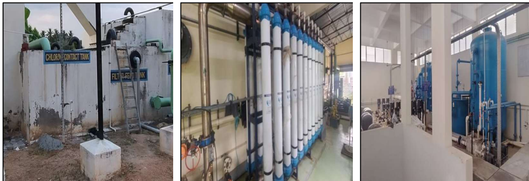
Figure 2.11: Photographs of Tertiary Treatment Units installed in STP
