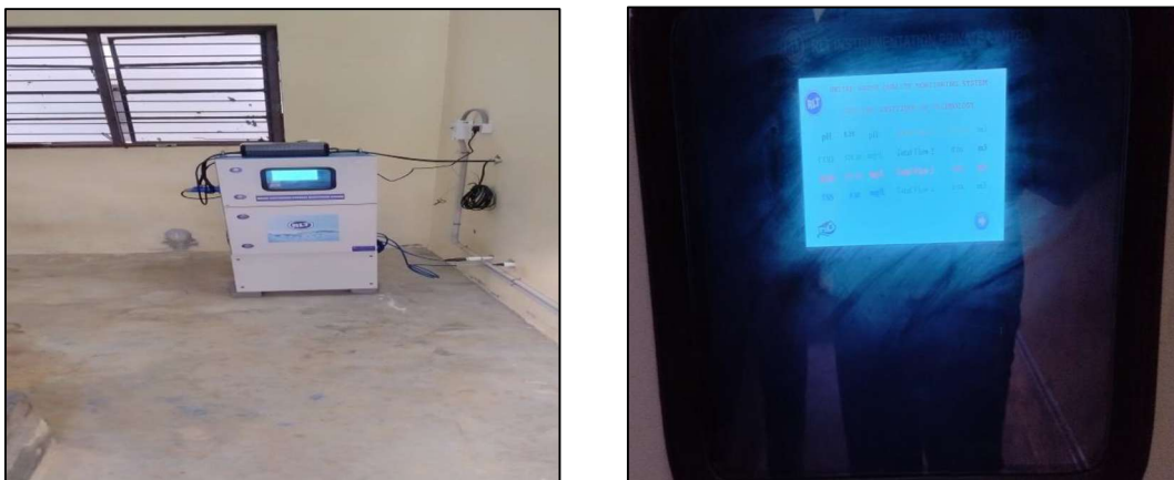
Figure 2.12: Photographs showing OCEMS installed at the outlet of STP
