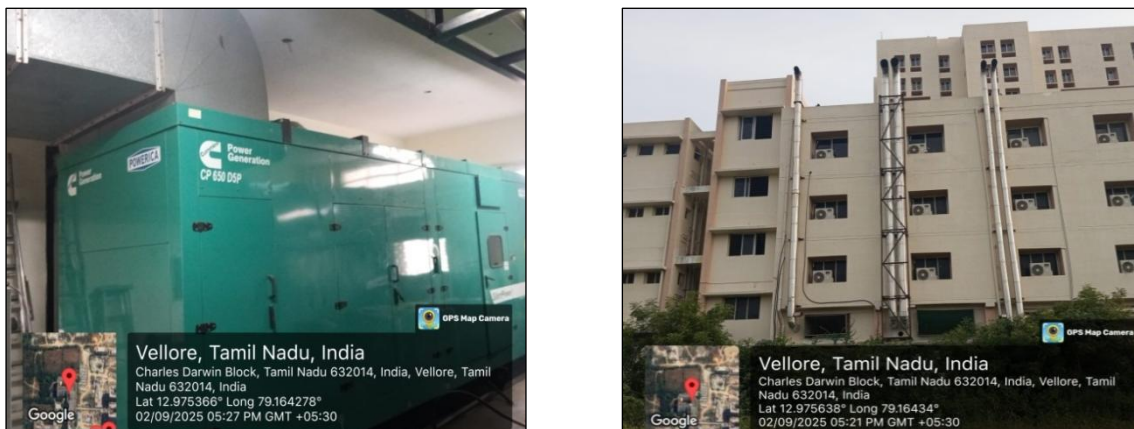
Figure 2.22: Photograph showing DG Sets provided with acoustic enclosure and stack height as per CPCB norms
