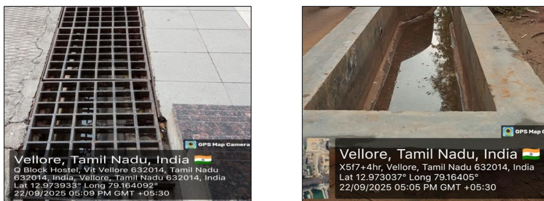
Figure 2.14: Photographs of Storm water drain
