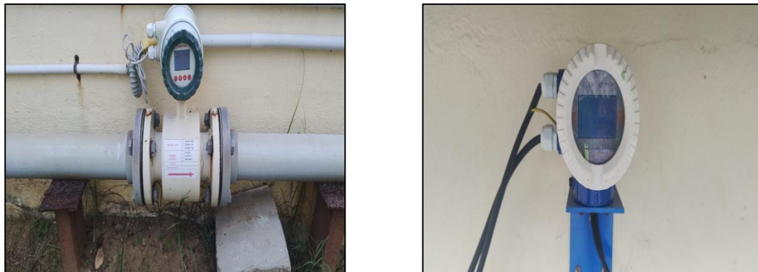
Figure 2.10: Photographs of Water meters installed towards monitoring total water consumption.
