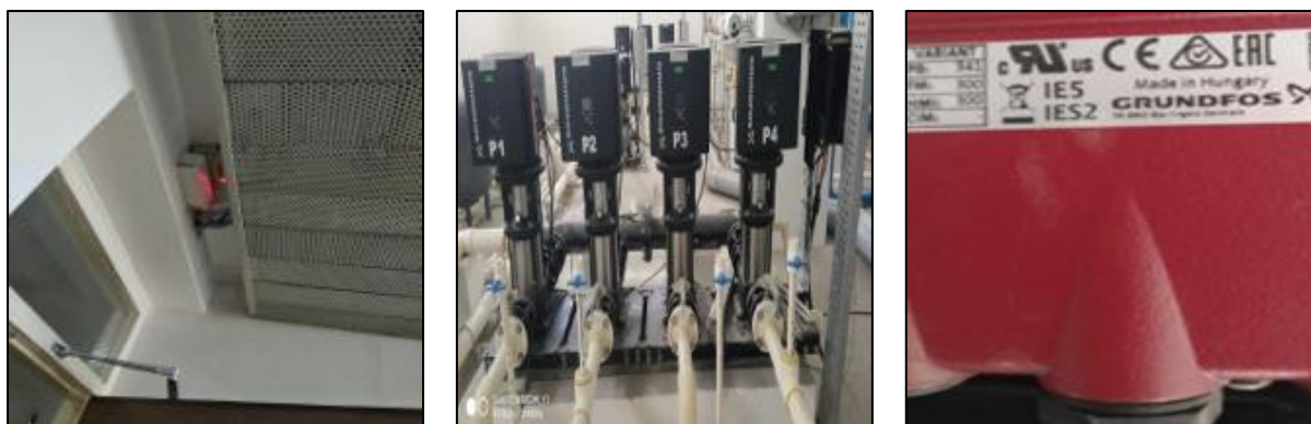
Figure 2.6 Photographs showing energy saving machines installed in the institution
