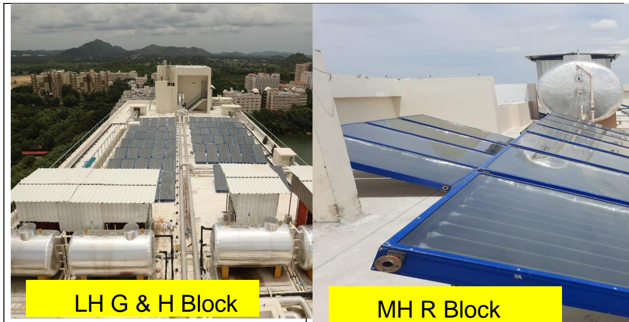
Photographs 27: Solar Water heater with heat pump - VIT,Vellore
