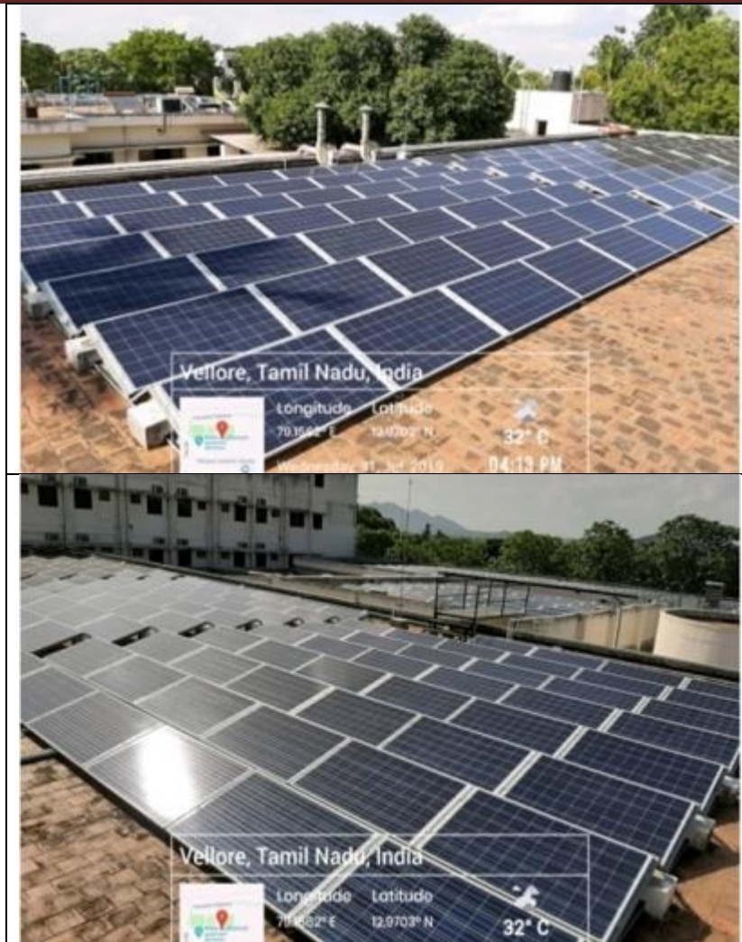
Photographs 16: View of Solar Panels – VIT, Vellore
