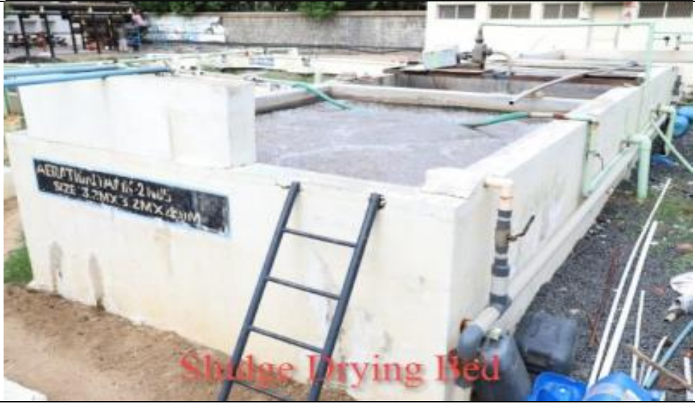
Photographs 22: View of Liquid Waste/Sludge Treatment Plant - VIT, Vellore
