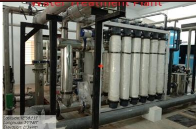
R.O.Plant for Drinking water supply
