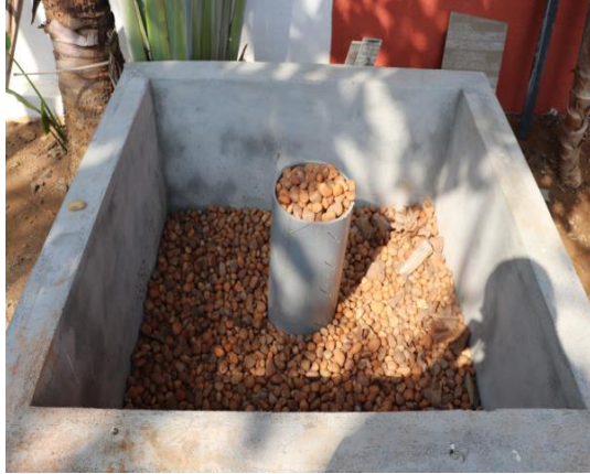
Fig.1 – Rainwater Collection Pit
