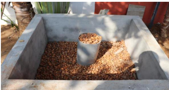
Rainwater Collection Pit
