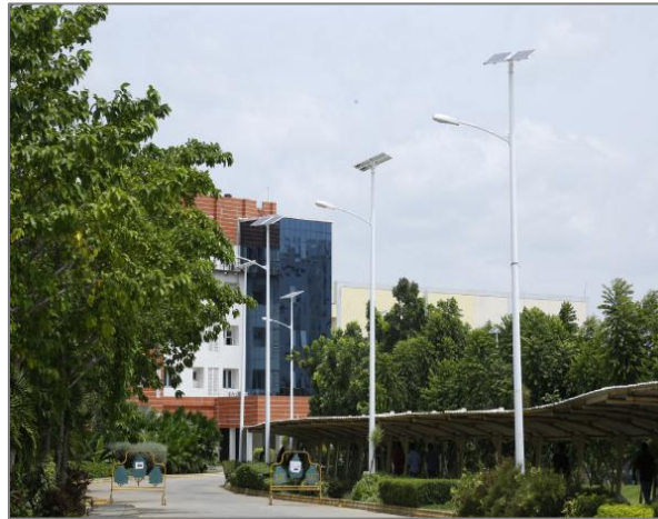
Solar panels powered exterior (pathway) lightings
