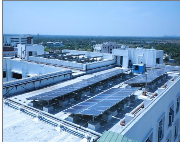
Solar Panels installed at the Roof-tops of the building
