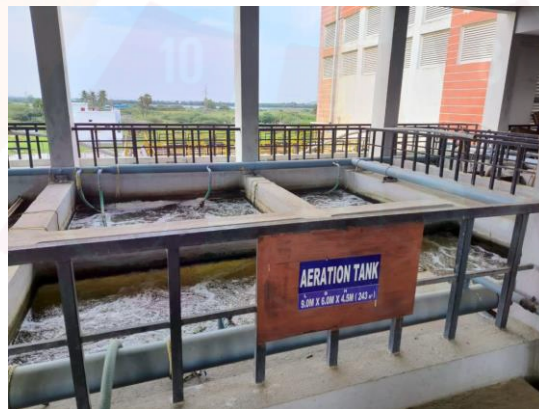
Sewage Treatment Facility (STP) at VIT Chennai
