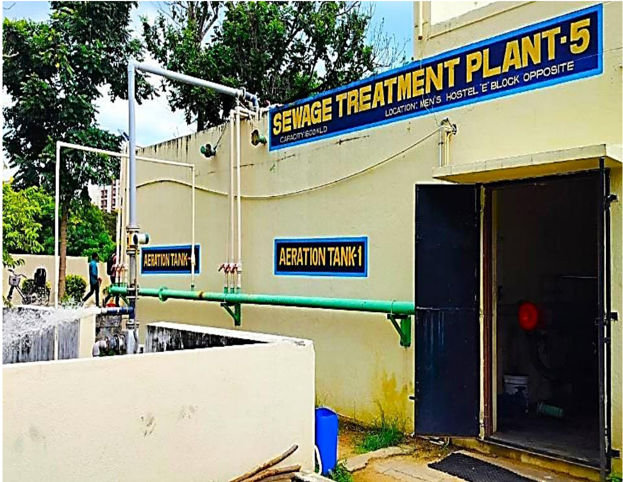
Preventing water system pollution
