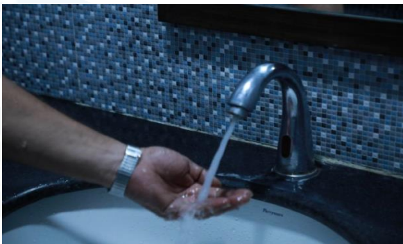
Power water saving through sensor based water taps
