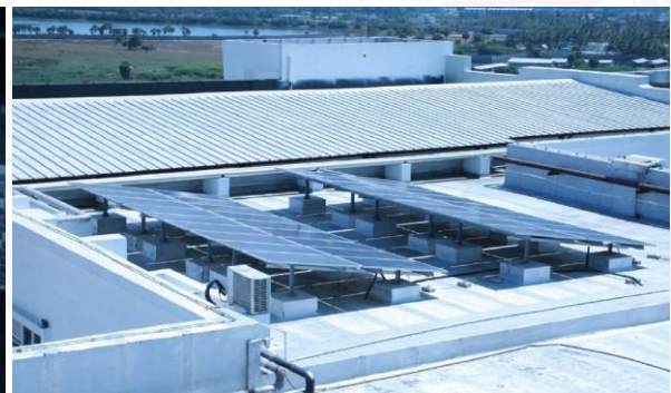
550 kW rated solar panels installed at roof top
