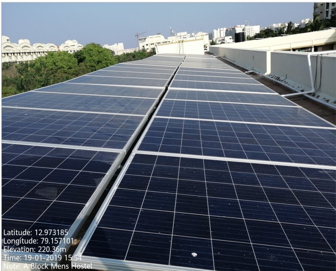
Latitude: 12.973177 Longitude: 79.164307 Elevation: 230.94m Time: 19-01-2019 16:26 Note: Solar PV
